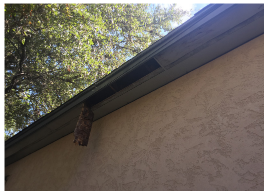
Likely wood rot needing attention
